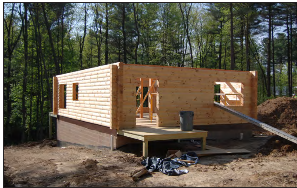
One of the ten rental cabins under construction at Pleasant Hill State Park
