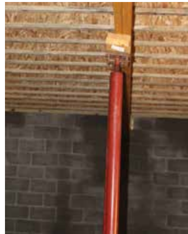
A post with a few blocks holding up the large post upstairs
